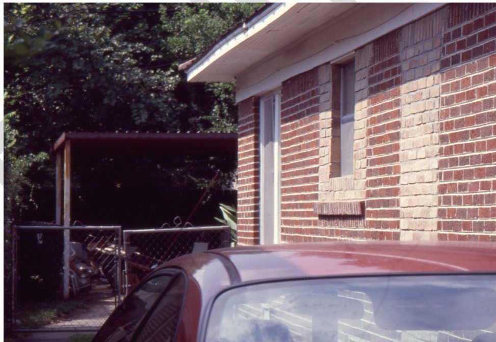
Figure 1 & 2 - Previously Filled in Door and Partially Window on Left Side, Images from 2012
